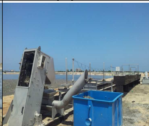
Khanyounis Wastewater Treatment Plant
